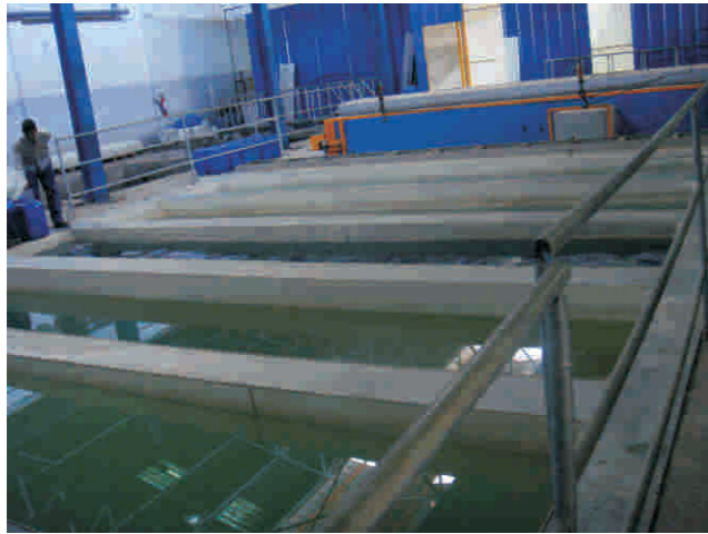
Immersion tank pretreatment system
